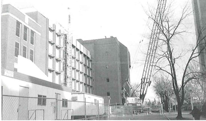
View of Fulmer Hall construction from Stimson Hall. Old Fulmer Hall is on the left, Fulmer Annex in the middle and the new SYN building is to the right.
